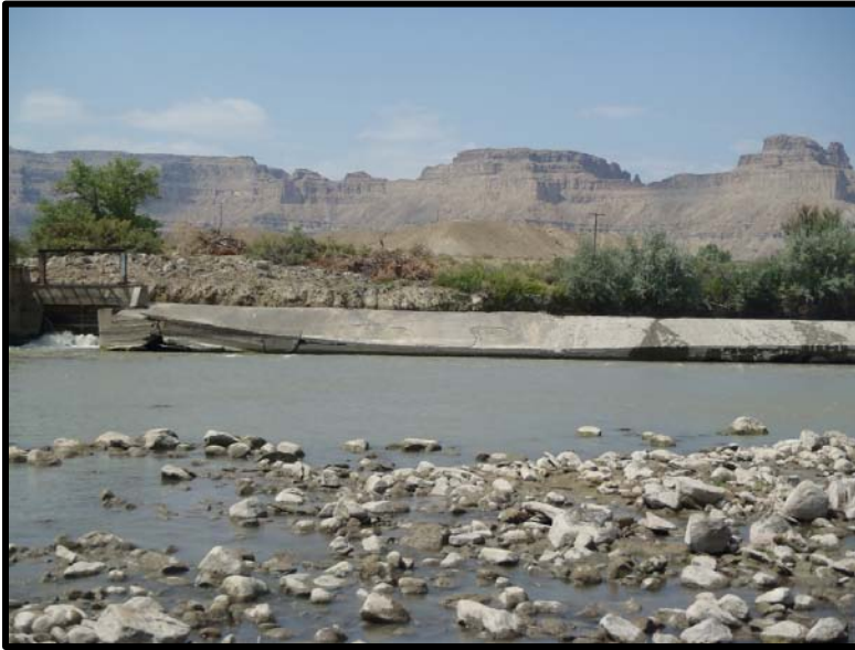
Damaged Concrete on West Side of Diversion.
