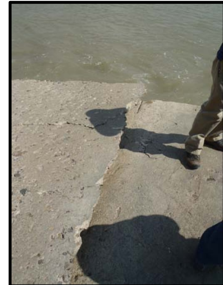
Damaged Concrete on West Side of Diversion.
