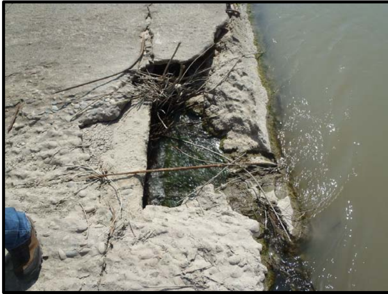
Damaged Concrete on West Side of Diversion.
