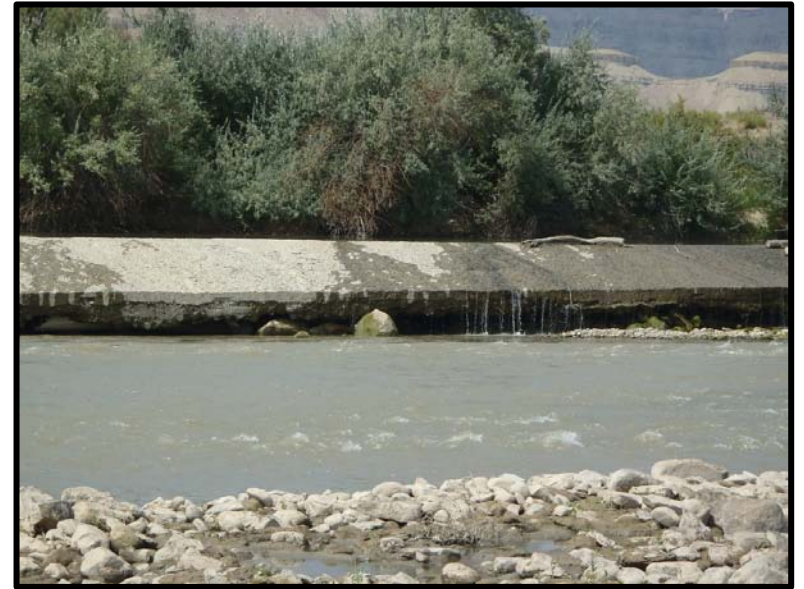
Undercutting on West Side of Diversion.
