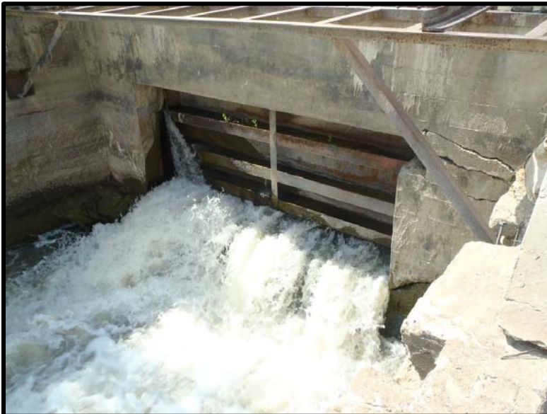
Damaged Concrete on Low-Level Slide Gate.
