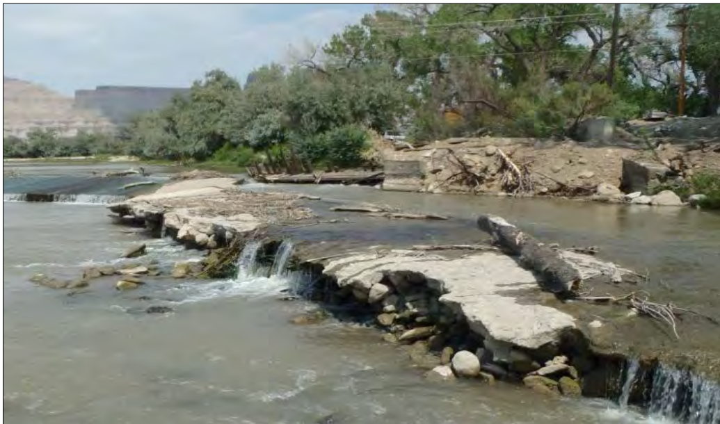
Picture 2-4. Damaged Diversion Structures, East Side
