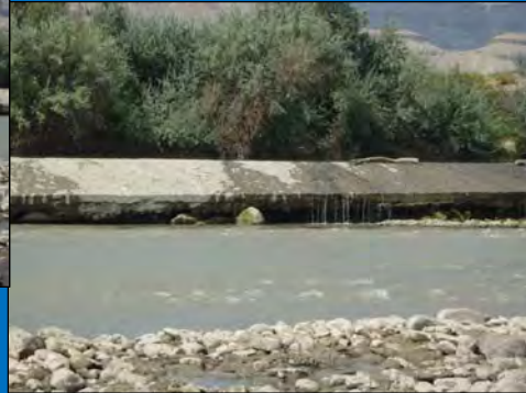
West End of Diversion Damage to Diversion Dam (looking u/s)
