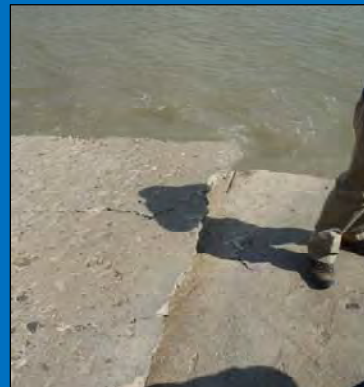
Damage to Concrete West End of Diversion
