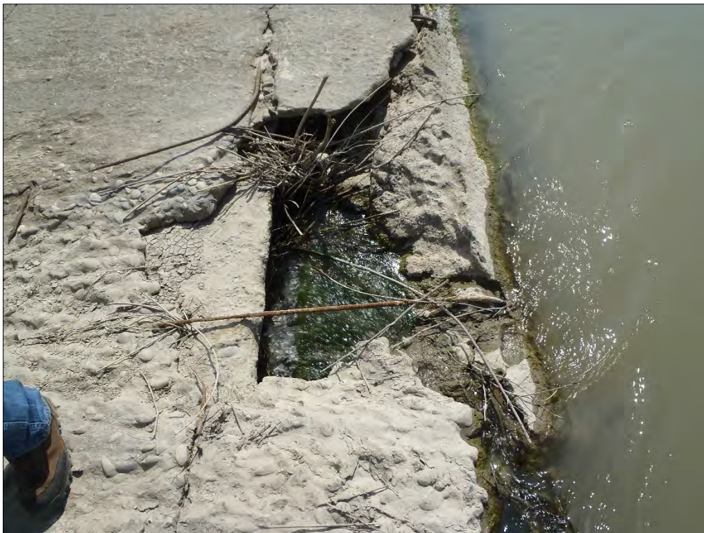
Picture 1-3. Example of Damaged Area
