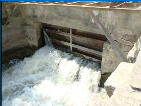
Damage to Slide Gate West End of Dam (looking u/s)
