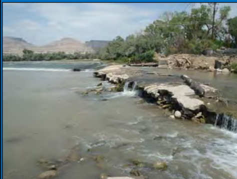
East End of Diversion Damage to Waterwheel Raceway (looking u/s)
