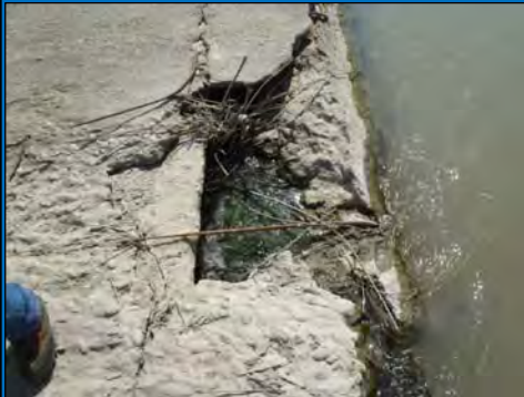
Damage to Concrete West End of Diversion
