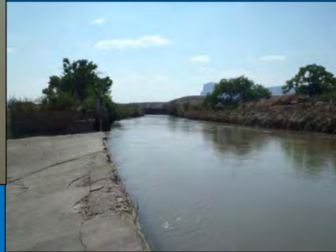
Damage to Concrete and Entrance to Raceway West End of Diversion
