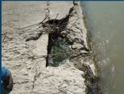
Damage to Concrete West End of Diversion
